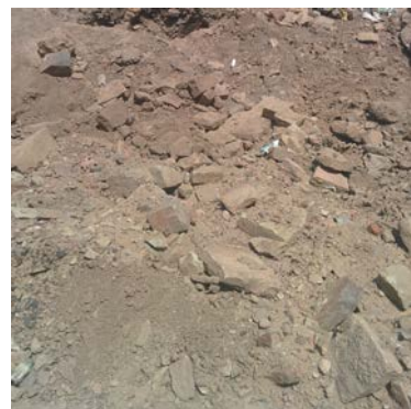
Figure 2. Loose soil and boulders at base of excavation
