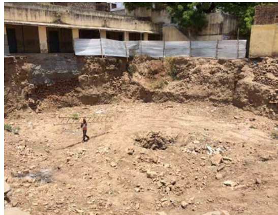
Figure 1. Excavation to 4 m depth showing loose heterogeneous boulders and stones in a soil matrix
