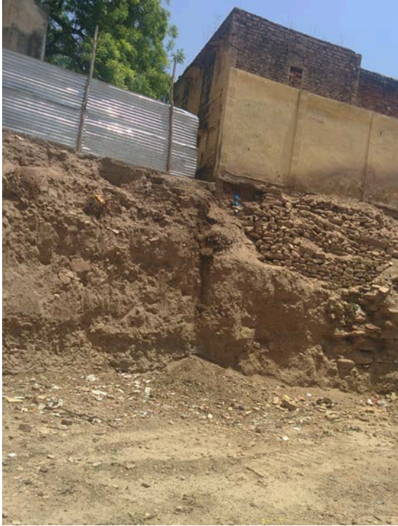
Figure 3. Steep excavated slope of the boulder fill adjacent to nearby existing building
